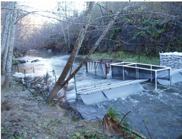
A weir was installed near the mouth of Prairie Creek. Photos by M. Sparkman.
